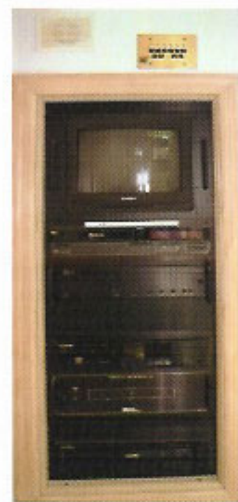
Sensitive audio/video components like the laserdisc player and surround sound processor reside in a rack outside the poolhouse where they are unharmed by moisture.
