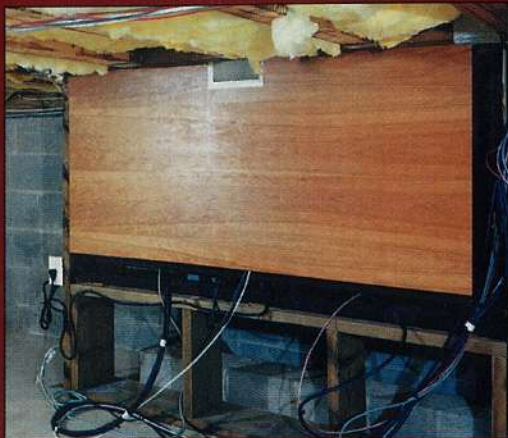
To mobilize the plasma, EDG called on Electrokinetics to build a double rack-and-pinion lift to support the display and center-channel speaker
