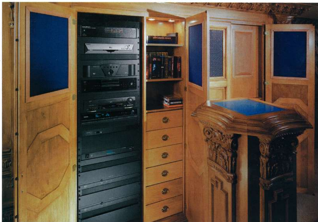
A custom cabinet housing the electronics preserves the magnificent theater’s design integrity.
